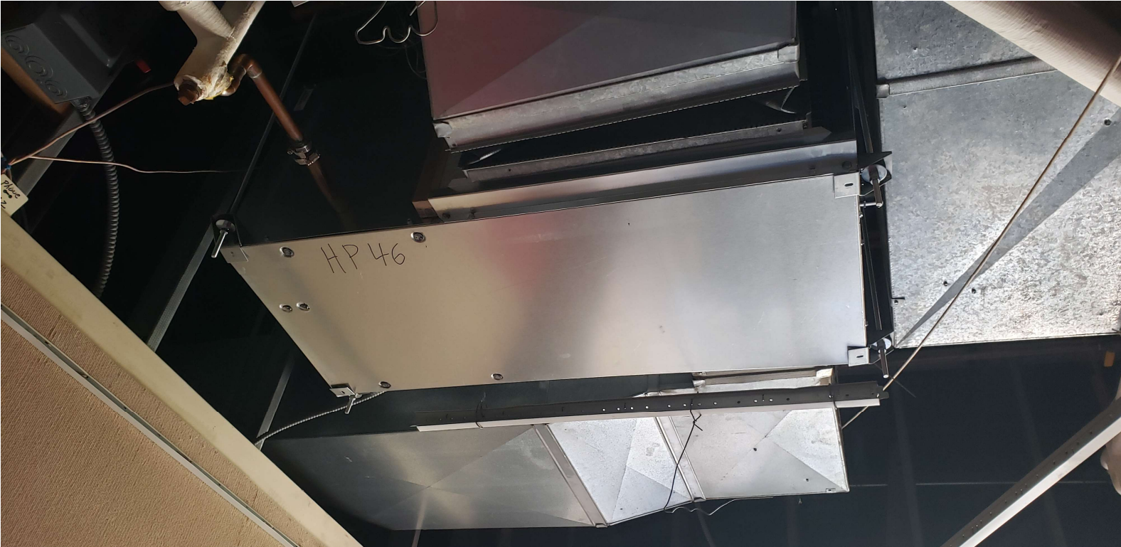
New heat pump installed
